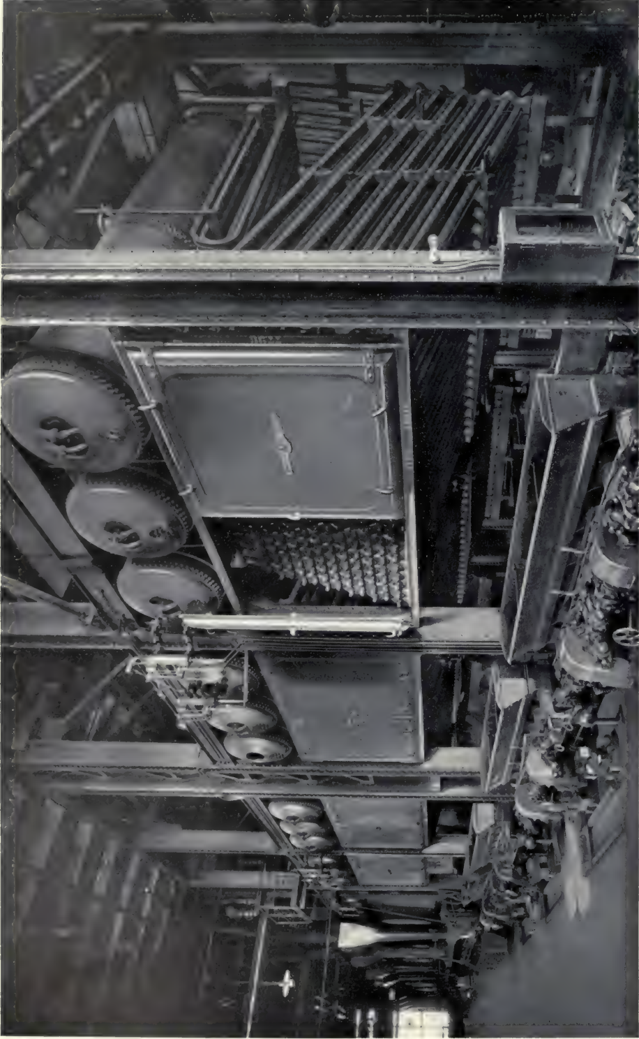
PENNSYLVANIA RAILROAD CO., LONG ISLAND CITY, N. Y., POWER STATION. 18,700 HORSE POWER OF BABCOCK & WILCOX BOILERS, EQUIPPED WITH BABCOCK & WILCOX SUPERHEATERS INSTALLED IN THIS PLANT. THIS COMPANY HAS BABCOCK & WILCOX SUPERHEATERS INSTALLED IN 31,800 HORSE POWER OF BABCOCK & WILCOX AND STIRLING BOILERS
